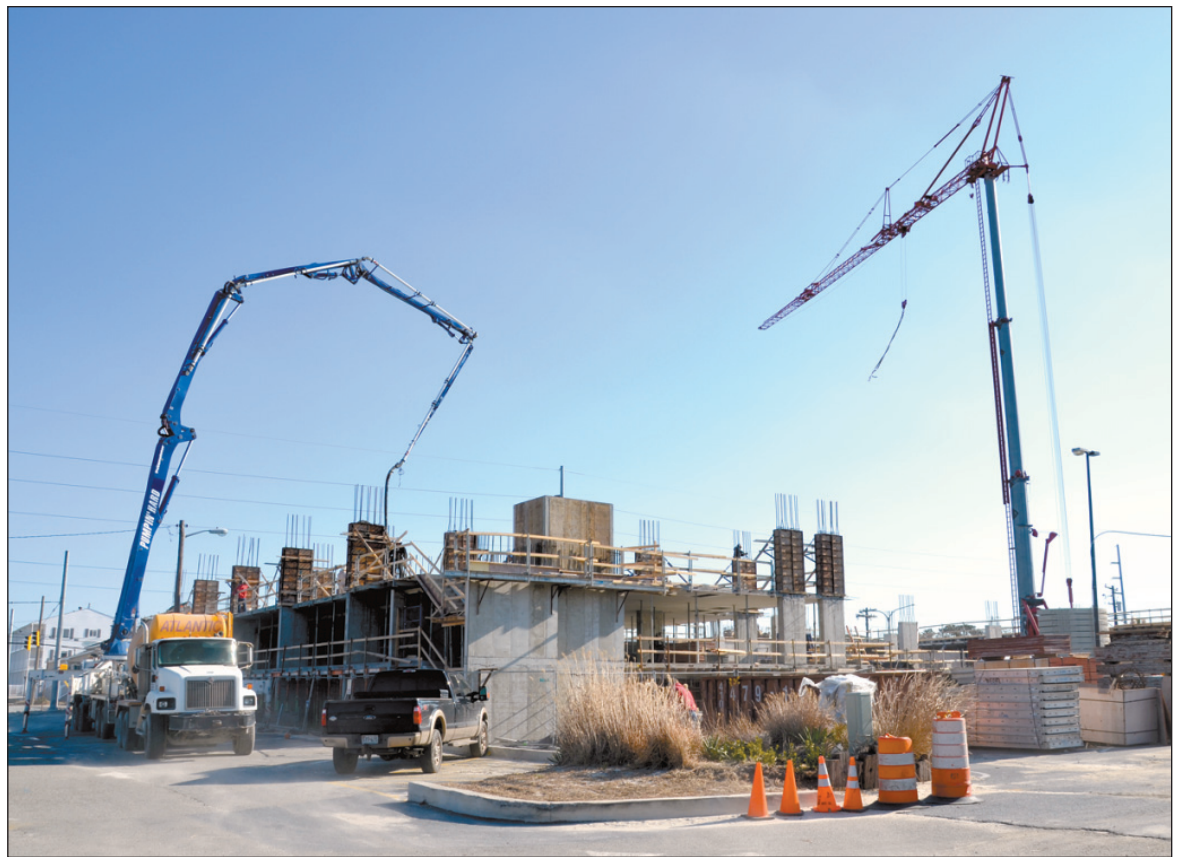
CONSTRUCTION WORKERS secure second-level columns for the third floor. The third-floor structure was completed in early January. Framing for the first set of Hyatt Place hotel rooms also started in early January.
